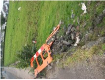
Pavement collapse into field
