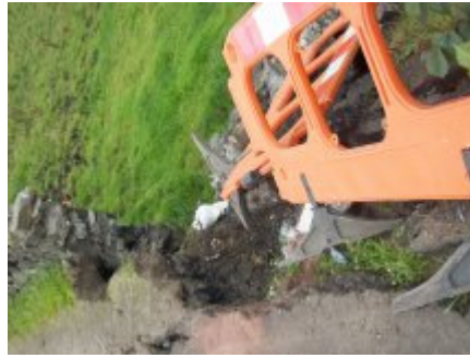
Broken wall/collapsed pavement
