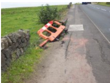
broken wall into field & collapsed pavement section
