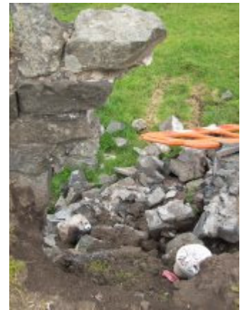
Broken wall/collapsed pavement
