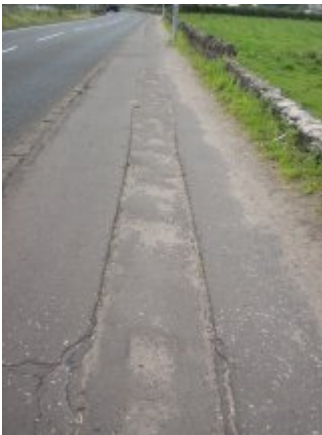
Poor surface which floods
