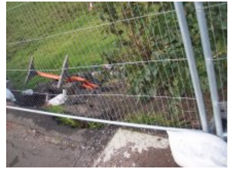
Fencing covering collapsed pavement
