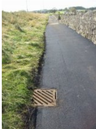
Drain cleared/installed at new section of pavement surface on approach to school
