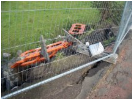
More collapsed pavement and fencing
