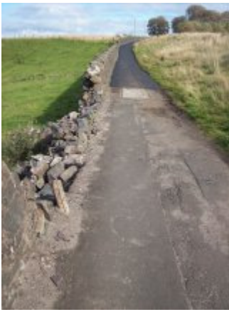
Looking towards the school section not upgraded at broken wall
