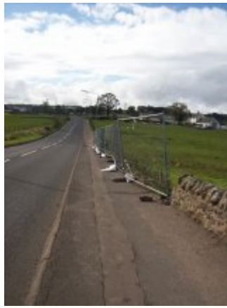
Fencing covering biggest gap in wall and collapsed pavement
